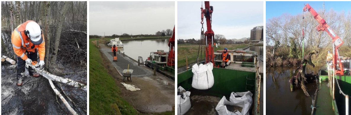
Riverbank tree work on the River Ant; path surfacing at Berney and Cantley moorings; removing a large tree trunk in the channel at Rockland Broad
