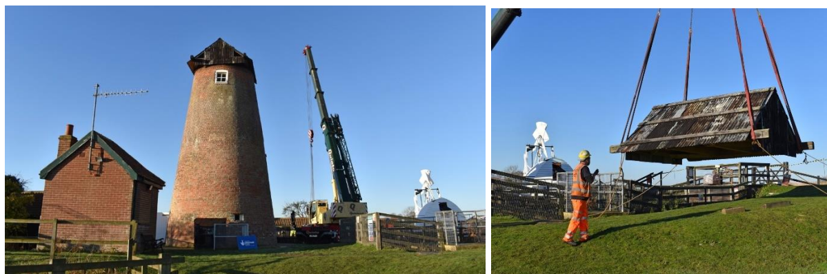
Stracey Arms Mill with its temporary roof being removed prior to fitting of the new cap
