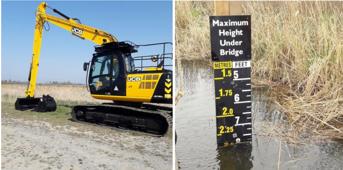
New JCB 180 excavator and One of the new gauge boards near Ludham
