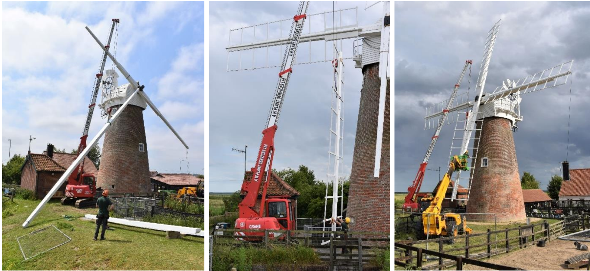
Crane lifting stocks & sails for fitting to the mill All images © Norfolk Windmills Trust
